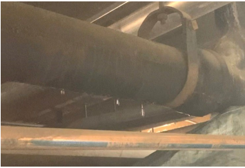
Dripping water from cracked cast iron pipe before being replaced using a Trust Fund grant.
